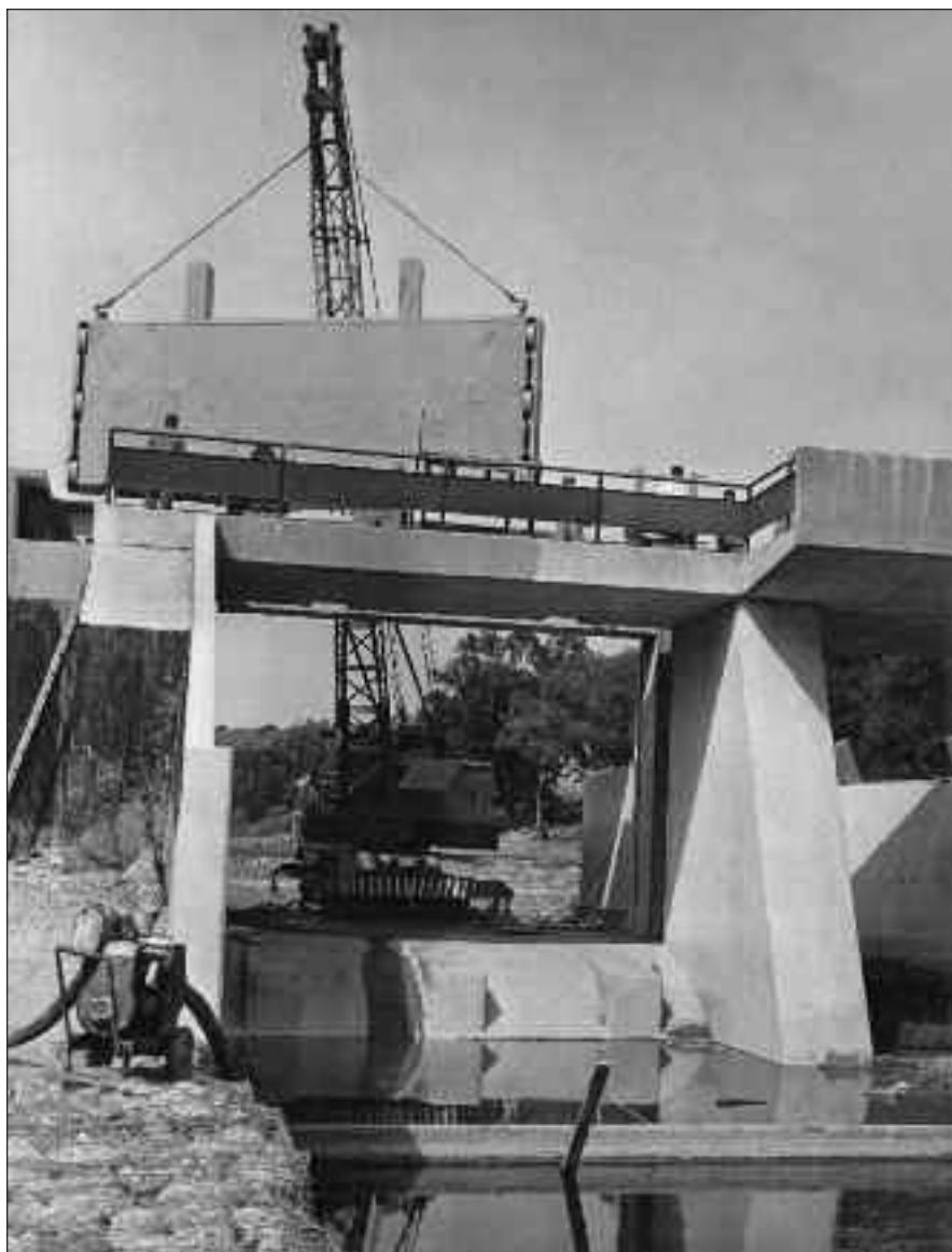
3046 A crane lifts a control gate into place during construction of the new Mitchell dam in 1964. The view is from south (downstream) of the dam.
