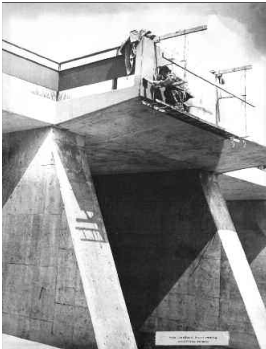
3045 A worker applies some finishing touches to the downstream face of the new Mitchell dam in 1963 or 1964. The photo is from southwest (downstream) of the dam.
