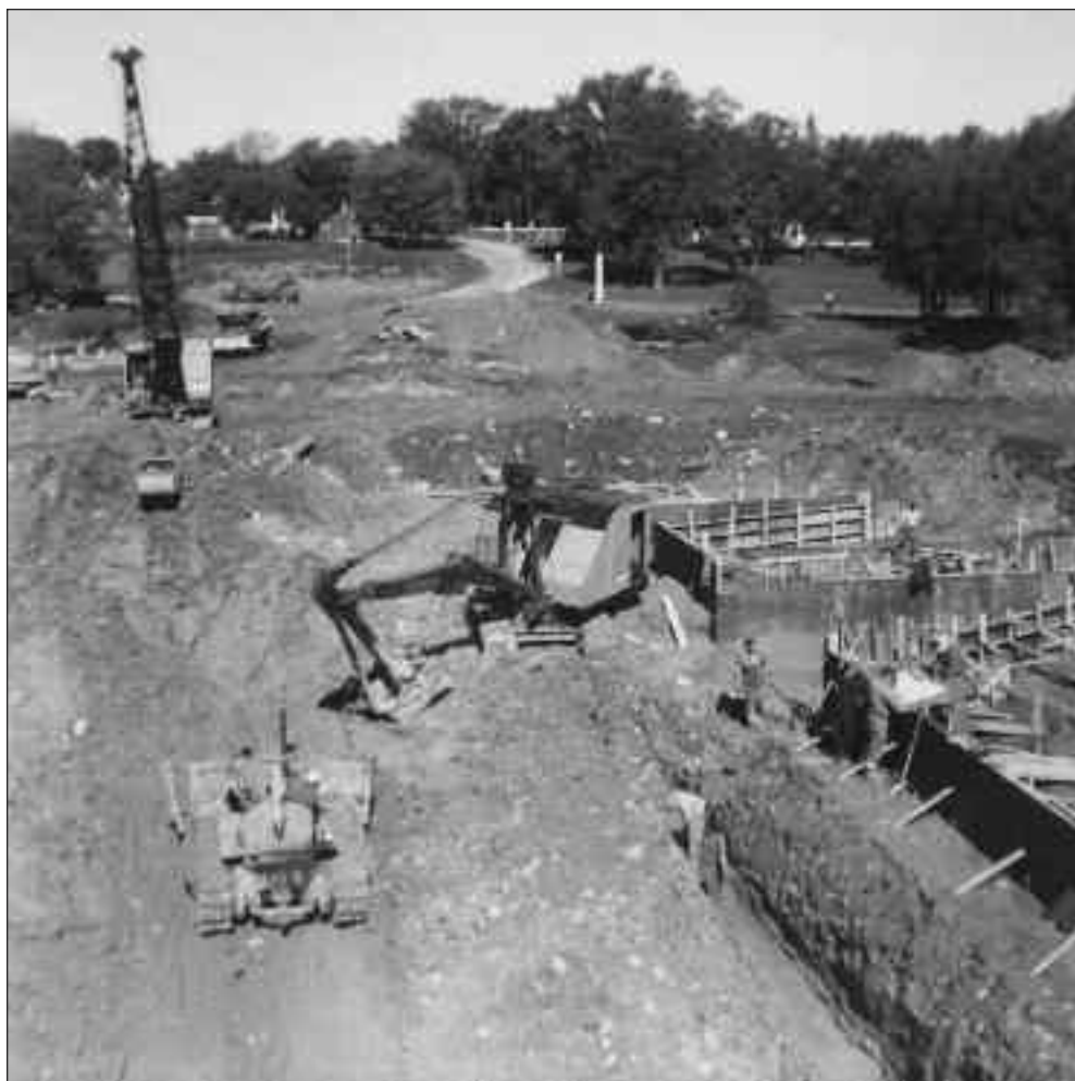
3040 A power shovel and bulldozer do most of the heavy work on the downstream side of the new Mitchell dam on the Thames River. The photo, taken in November 1962, is from the east side of the construction site, looking to the west, towards Blenheim Street.
