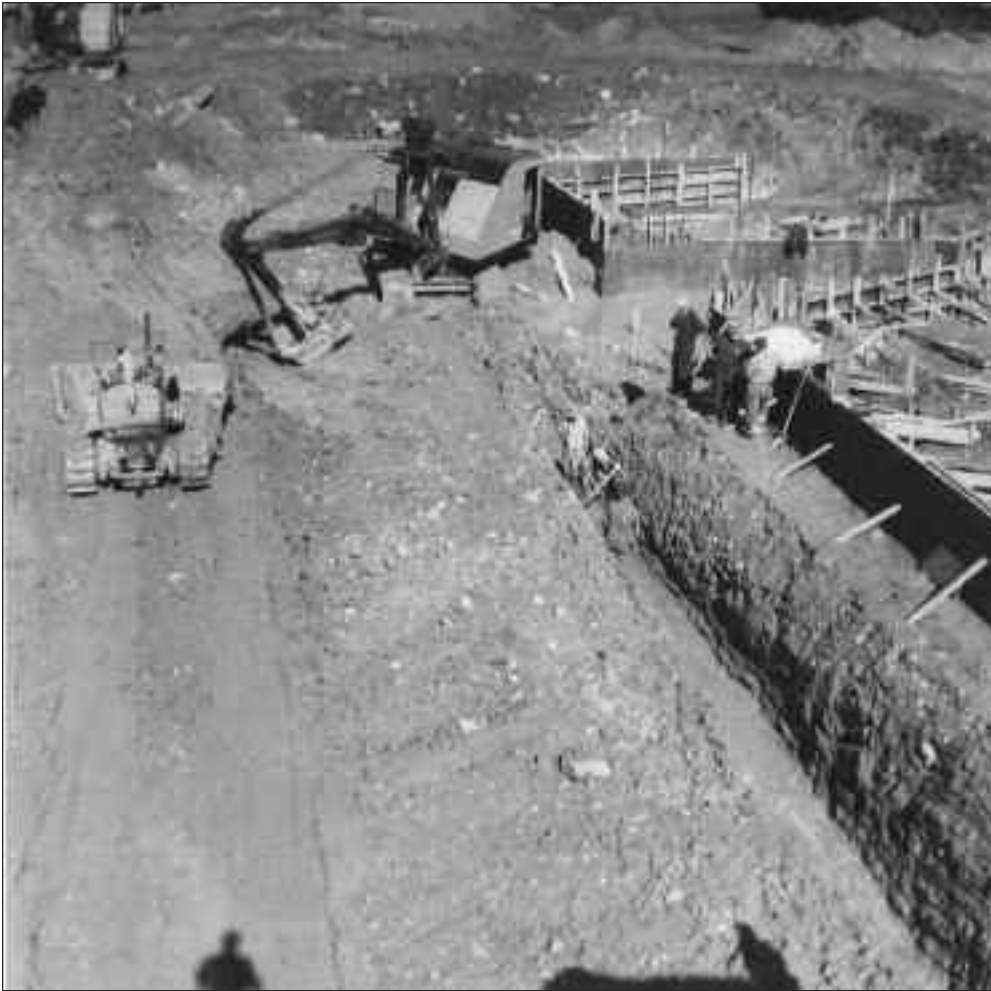
3041 Two power shovels and a bulldozer do most of the heavy work on the downstream side of the new Mitchell dam on the Thames River. The photo, taken in November 1962, is from the east side of the construction site, looking to the west, towards Blenheim Street and the Mitchell swimming pool.
