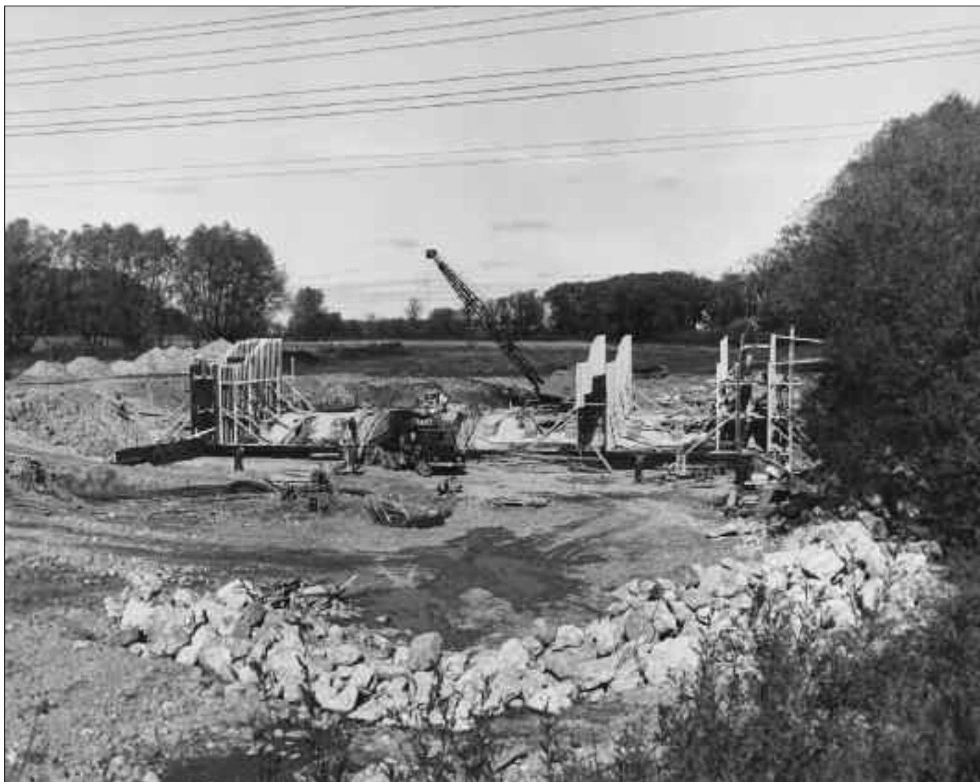
3043 A power shovel and a truck carrying concrete do most of the heavy work during construction of the new Mitchell dam on the Thames River in 1963. The photo is from south of the construction site, looking north.
