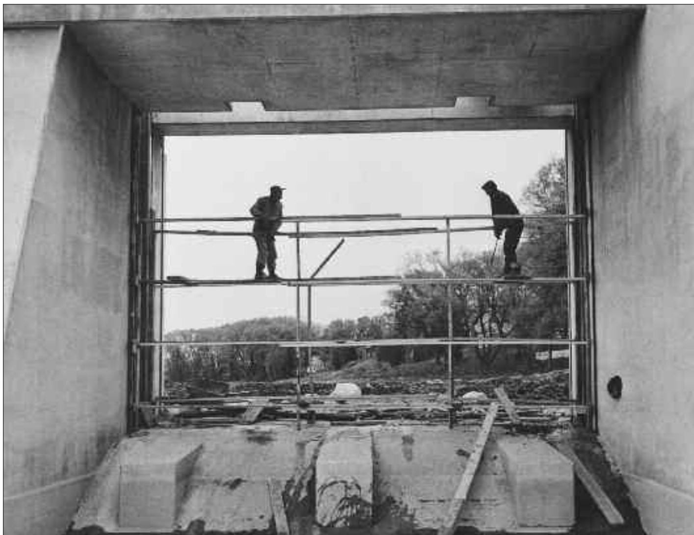
3044 Two workmen busy themselves in the spillway of the new Mitchell dam in 1963 or 1964. The photo is from south of the dam, looking north onto the Thames River bed.
